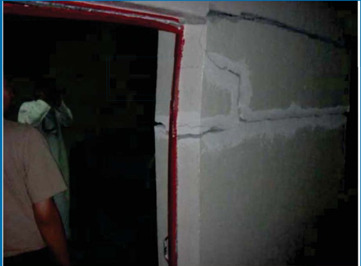
Reported damage around Masafi area (Al Shamsi, 2013)
