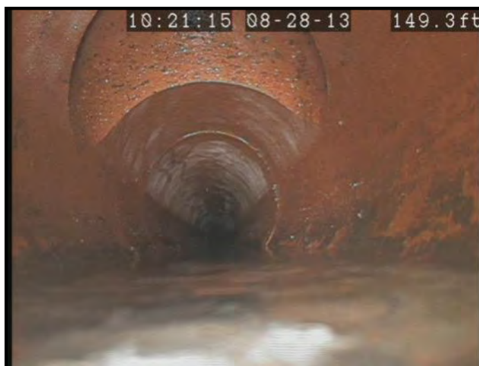
Figure 11: Photograph of 8" vitrified clay sewer pipe taken by MWCD sewer camera. Note the cleanout connection located at the top of the pipe. Photograph by Author.
