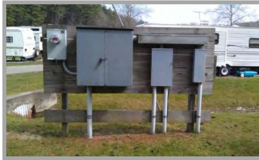
Electrical Junction boxes
