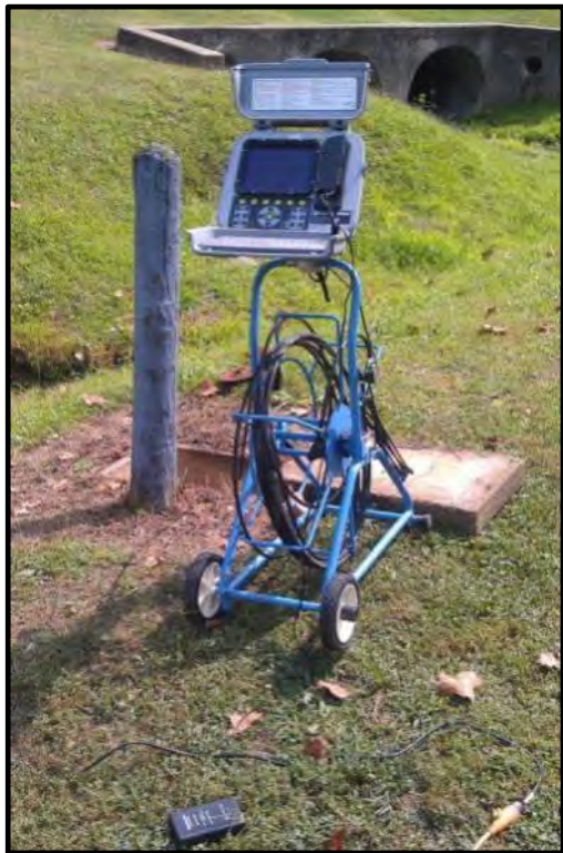
Figure 10: A push style sewer camera in use at a sewer cleanout in Tappan Lake Park. The video camera is linked to a laptop and able to collect images and video. Photograph by Author.
