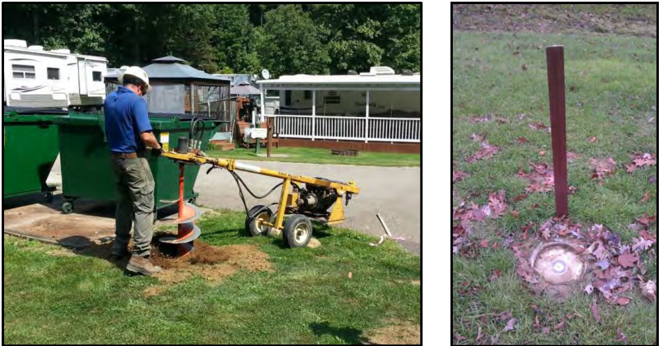
Figure 5: Left: Installation of survey control monument using a gas powered auger. Monuments were placed 42” deep to be below frost line. Right: Final product of monument and witness post. Photograph by Author (July 2013).
