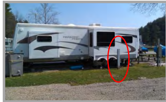
Electrical Pedestals at Campsites
