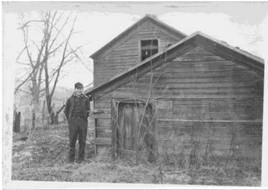
Figure 6 Damage to a dwelling in the Whitewater valley due to sedimentation. Photo Courtesy of the Winona County Historical Society.
